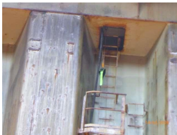
Figure 5: A safety belt with shock absorber and lanyard attached to a rope which is fixed on a hatch opening; the seafarer removed the safety belt to move down the fixed vertical ladder, before falling from a height of approximately 8 m to the cargo hold bottom and sustaining fatal injuries
